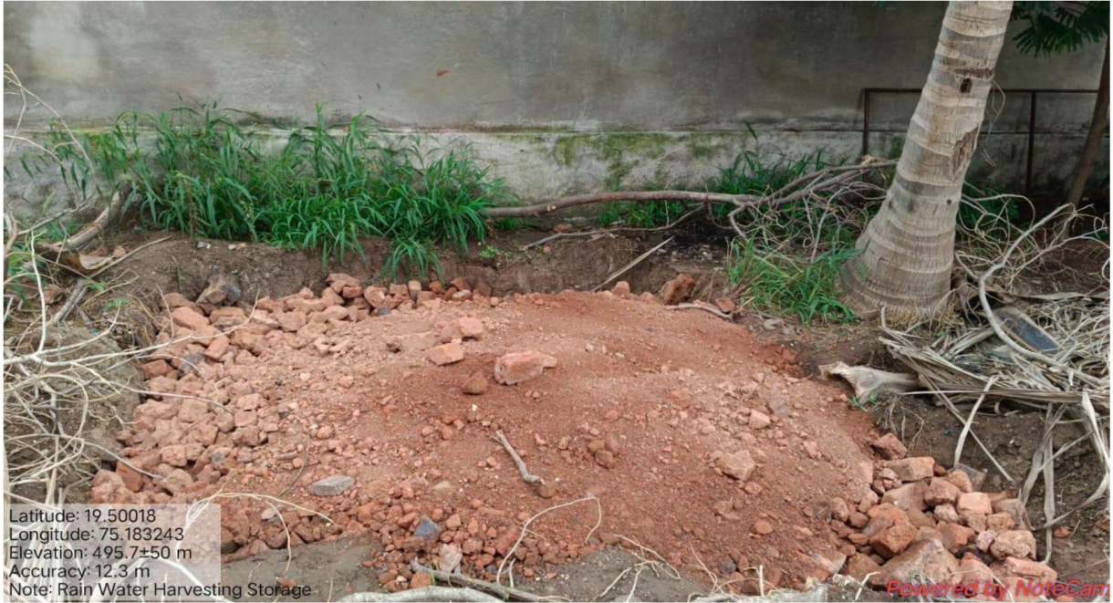
Rain Water Harvesting Storage.
