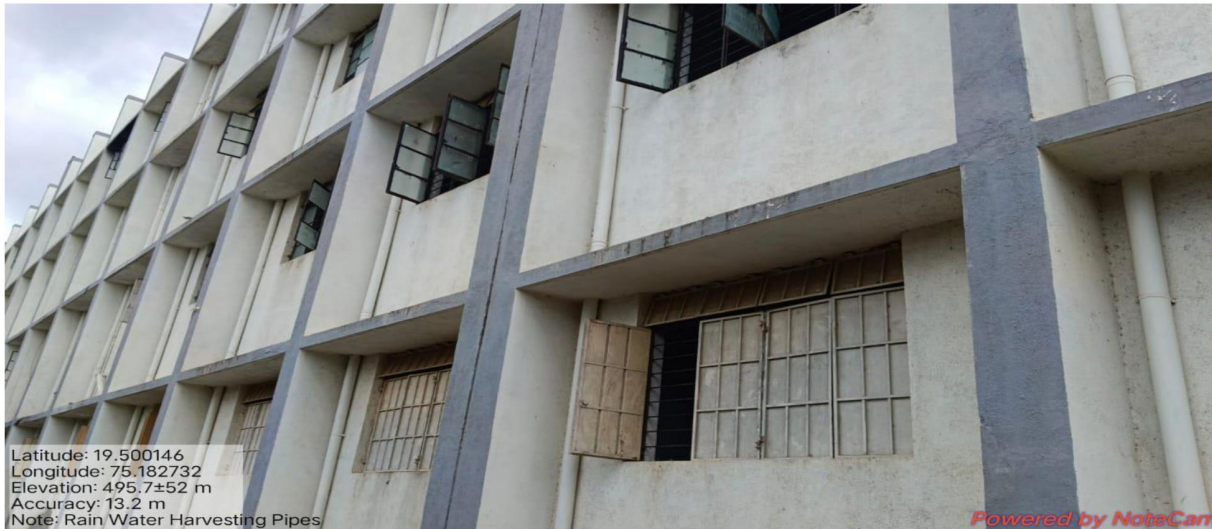
Rain water Harvesting Pipe
